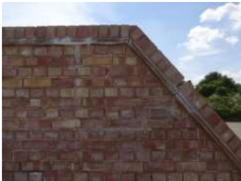
Example of TSA damage affecting the end wall of the new central spine in Fighter Pen KC12. Salt staining is also visible.
